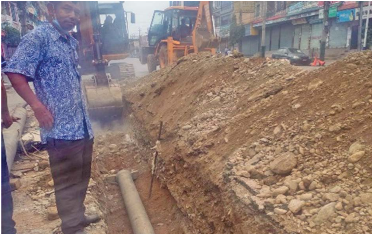
Photograph 12: 250mm DI Pipe Line Laying work From Srijana Chowk to Prithvi Chowk at Nepalganj branch
