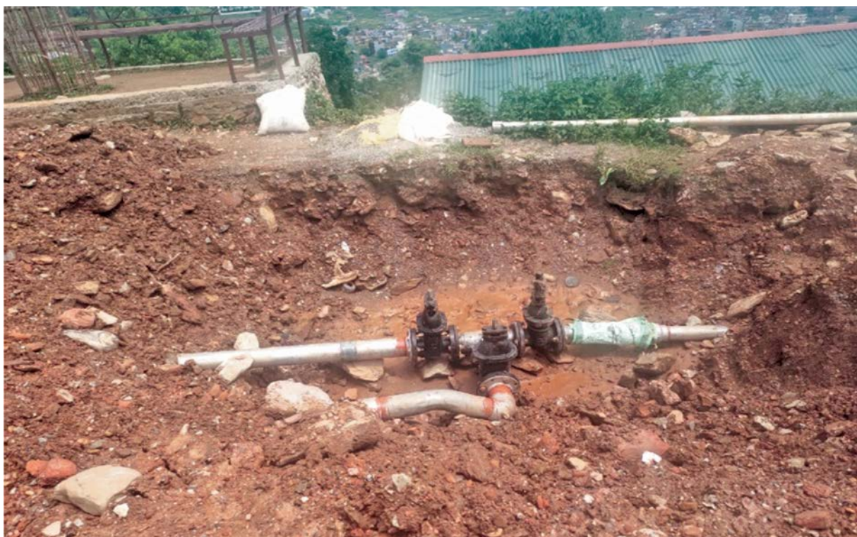
Photograph 13: 250mm DI Pipe Line Laying work From Srijana Chowk to Prithvi Chowk at Nepalganj branch
